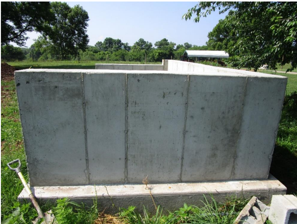
Photo 8 Outside face, north wall 6 weeks after forms were stripped. Note that much but not all of the discoloration is less apparent.
